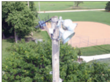
Figure 4. TVWS hotspot antennae serving Scott Street Ball Fields
