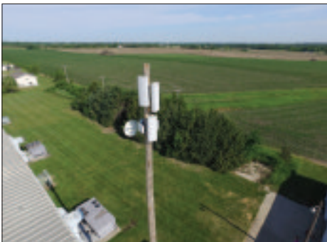
Figure 2. TVWS base station mounted on a 60-foot pole
